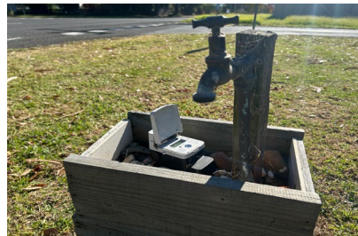
An example of a digital meter
