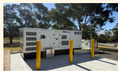
Back up generator
